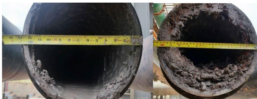
Figure 7. Scaling severity assessed in SCT discharge pipelines during brief shutdown
