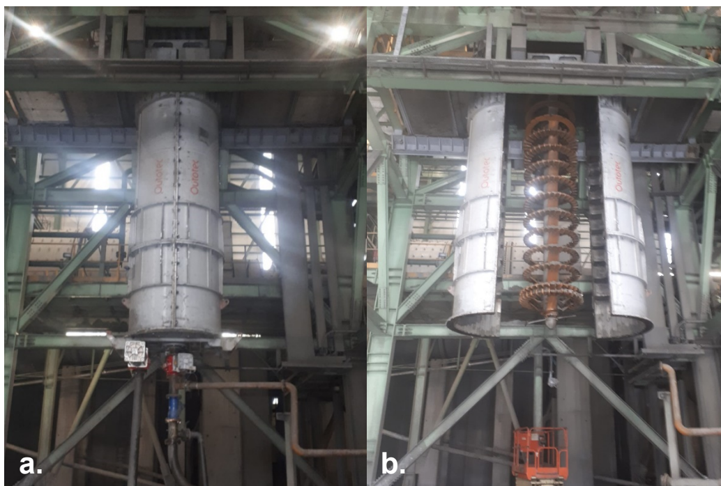
Figure 2. HIG mill at the copper mine.
