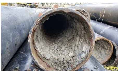
Figure 2. Scale deposited in pipe section
