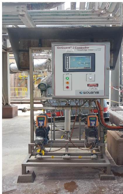
Figure 8. The Solenis OnGuard™ i Controller installed at the SCT circuit, PVDC
